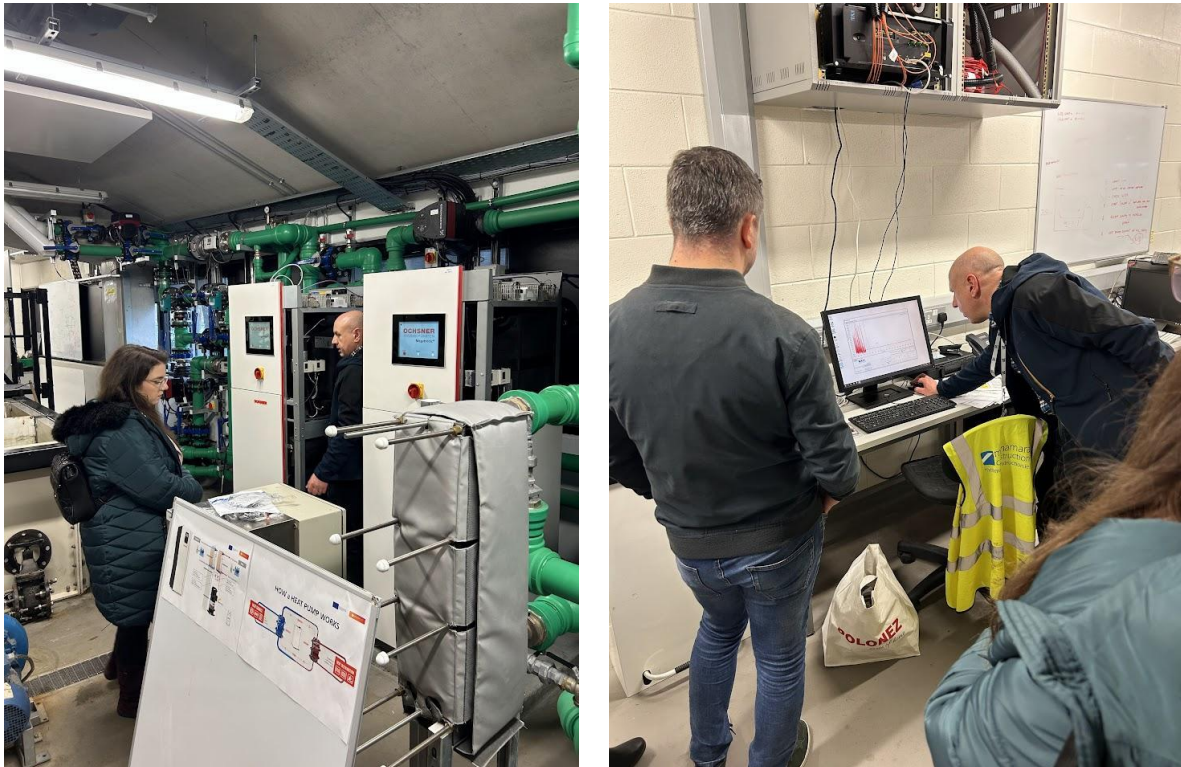
Figure 12. Heat pump plant with data demo from in Alice Perry building (with boreholes as the primary energy source)
